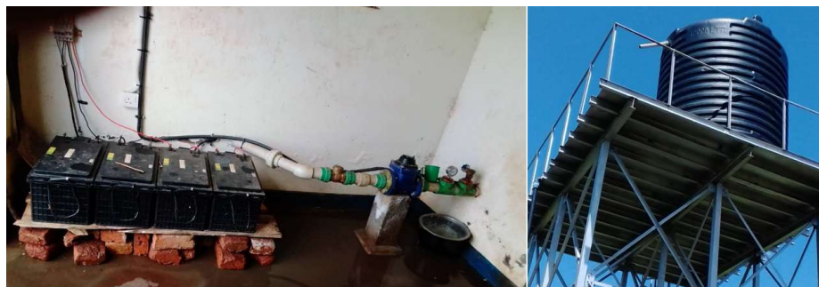
Figure 5-63: Current state of storage batteries and reservoir
