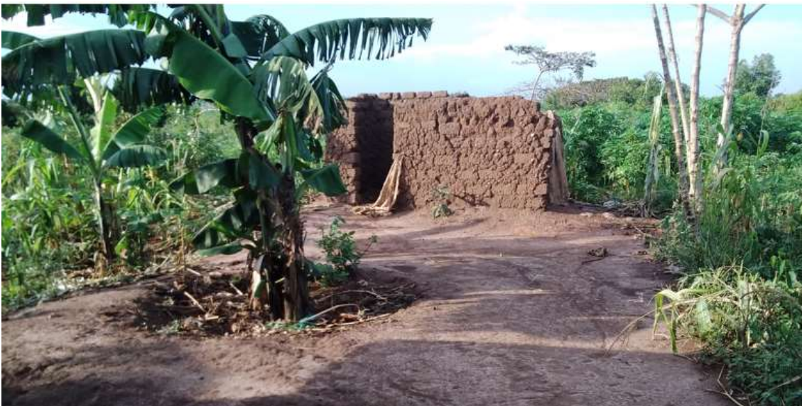
Figure 0-73: Poor pit latrine in Mutunda RGC
