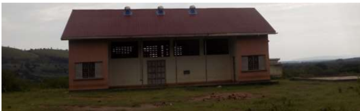
Figure 4-103: Un-used bulk store (constructed by CAIP programme with funding AFD) at Kikagati
