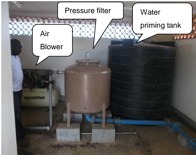
Figure 1-6: Pressure Filtration Unit & Water Priming Tank
