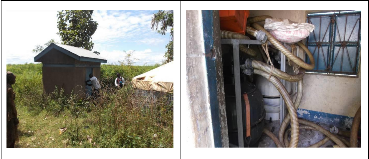
Figure 1-11: Pump House, disinfection tanks and flexible pipework in the Pump house
