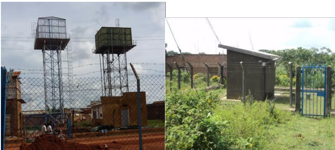
Figure 1-5: Reservoirs and borehole pump house for the existing Kaliro town water supply system
