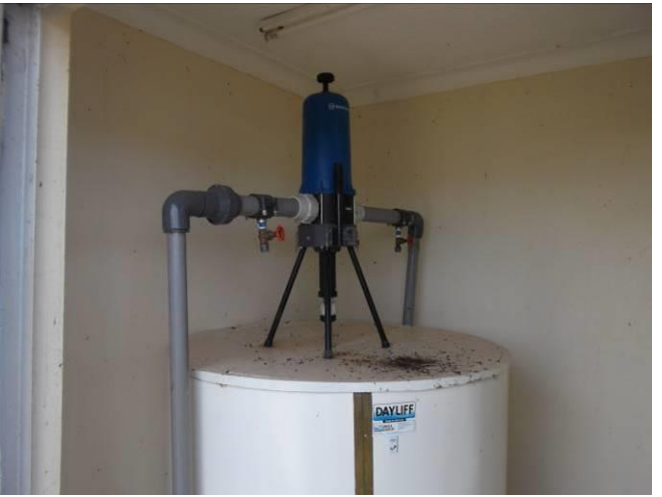
Figure 1-9: Chlorine Dosing Unit
