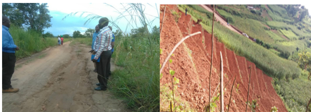
Staff of MWE conducting assessment of potential sites for flood control and water harvesting in Aswa Catchment; Showing a Flood control infrastructure in Maziba catchment
