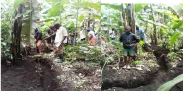
Community Members inspecting the construction of a Water Infiltration pits for harvesting run-off at a banana plantation in ukumbi cell
