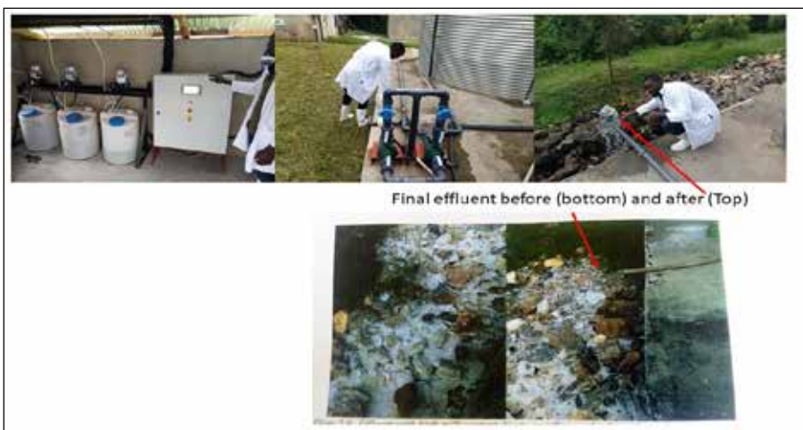
Top Effluent from dairy Company (GBK) after Wastewater Treatment Facility was Installed at GBK and bottom effluent before the Wastewater Treatment Facility was installed
