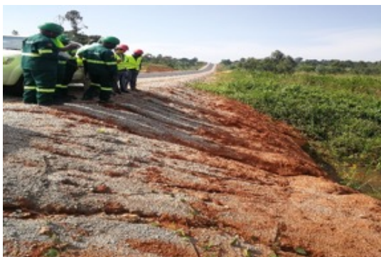
Poor Shoulder Management along the Mubende - Kakumiro - Kagadi Road
