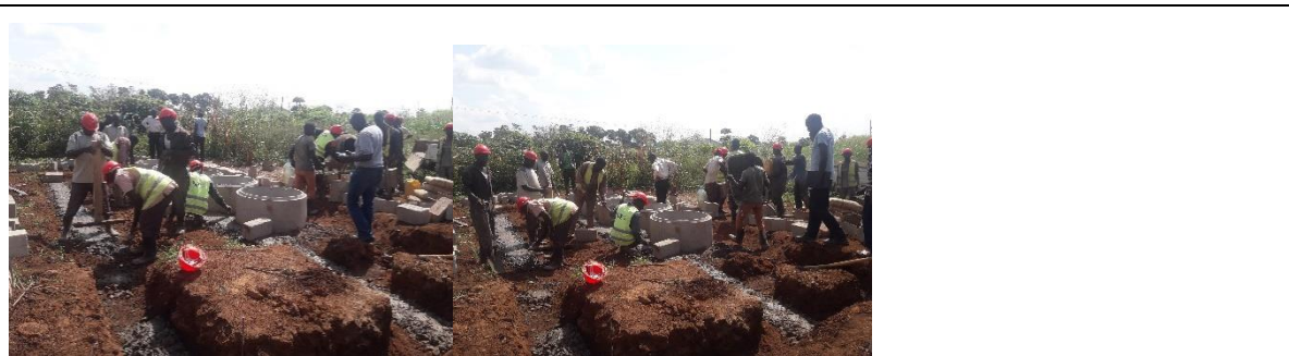
Construction of the substructure at Anyeke Health Centre III in Oyam District
