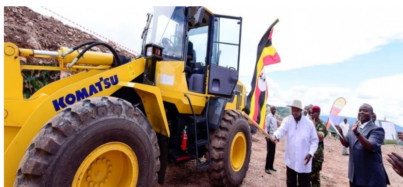
Ground breaking of Kikyenkye- Nyabuhikye Gravity Flow Scheme by H.E. President Yoweri K. Museveni and State of Minister for Water, Hon. Ronald Kibuule in Ibanda District
