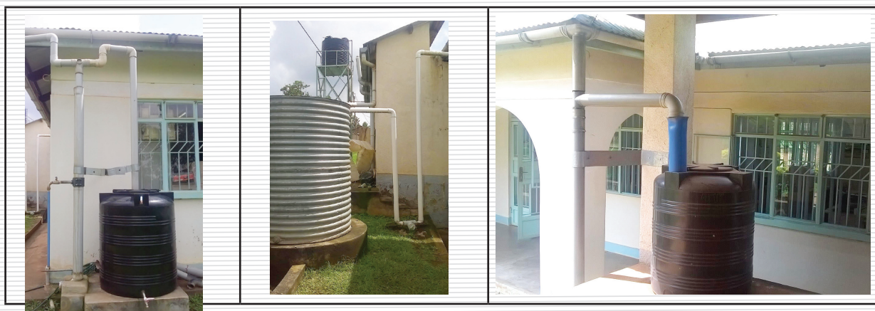
Figure 8: Different forms of first flush designs used in rooftop catchment to avoid the 1st dirty water of the rain (Photos from ATC)
