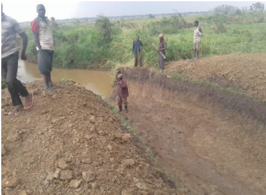
Photo 16: An un-planned diversion channel on river Manafwa for Rice irrigation in Butaleja
