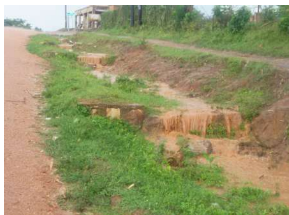
Runoff erosion in Lwakhakha
