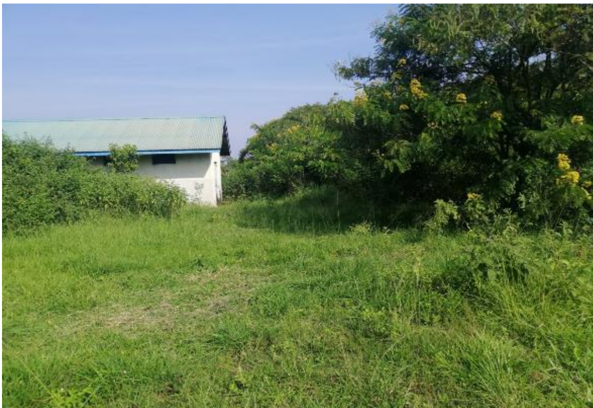
Plate 4.30: A pump house, the bushy part is the site where the incomplete tank structure is located
