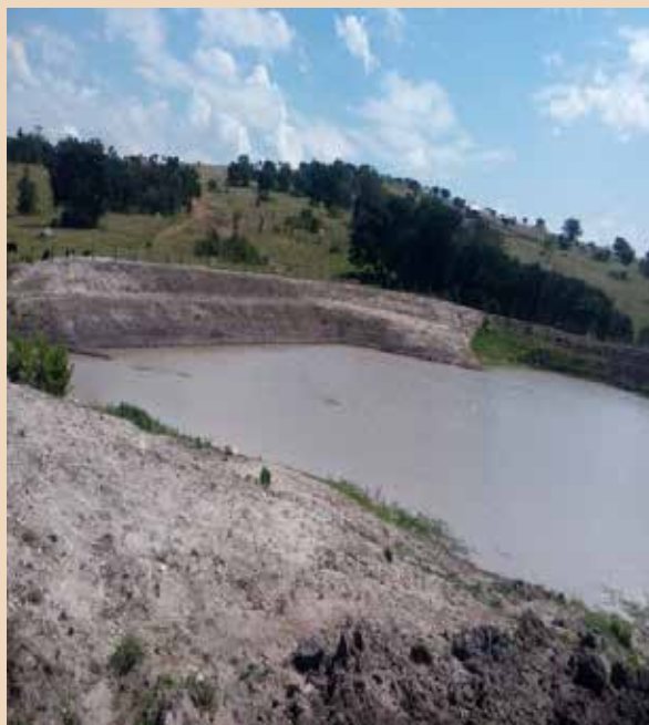
Canon George Mugisha valley tank constructed in Mbarara District
