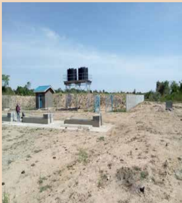
Cattle troughs, Storage tanks and a fenced water reservoir at Bamusuta Valley tank
