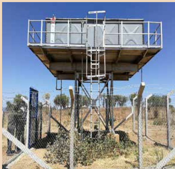
Functional water storage reservoir
