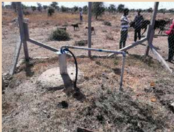
3.4 m 3 /hr yield borehole with submersible Grundfos pump
