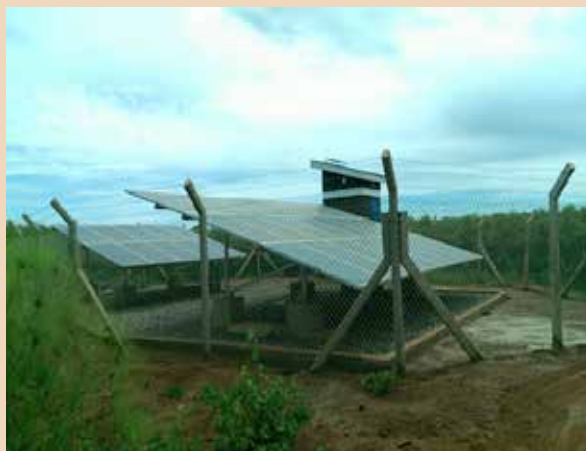
Fenced off Solar panels and a power house
