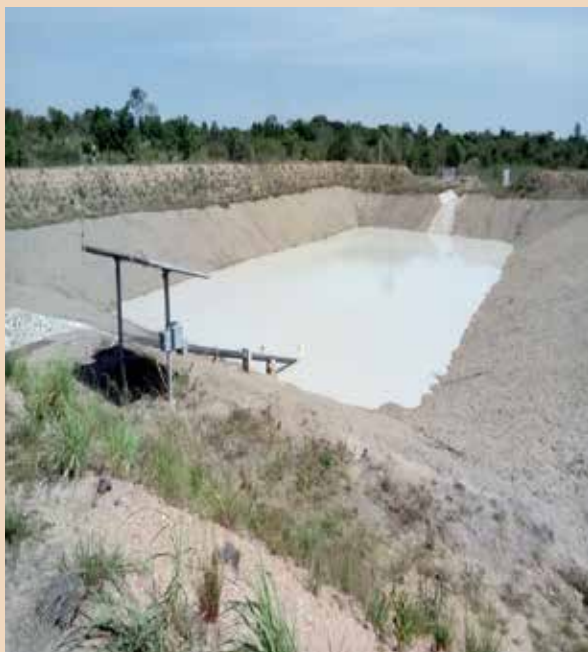
Solar Abstraction system and water reservoir at Lwenyana Valley tank in Nakasongola District
