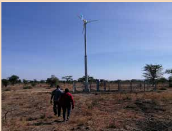
Windmill turbine was functional mounted on 12 m tower
