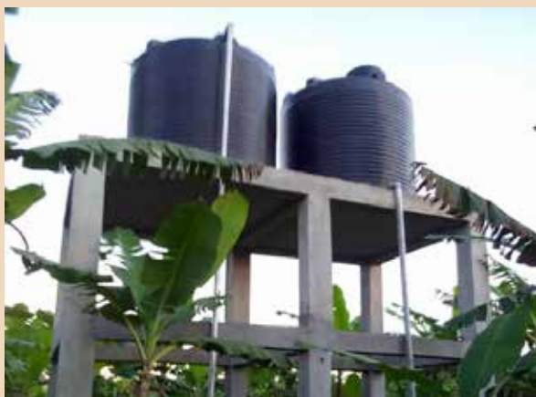
Tank Reservoirs for the Irrigation system
