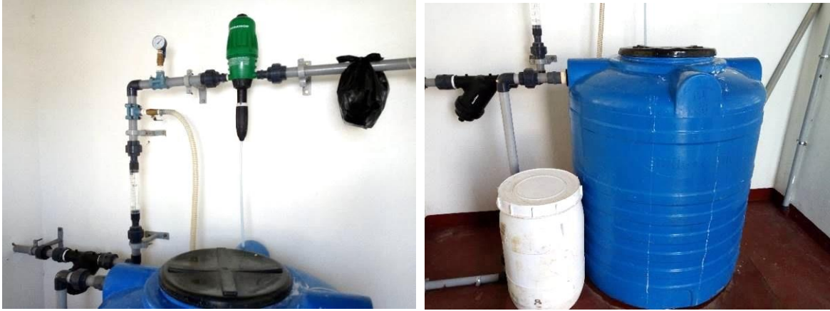
Figure 6-5: L-R Online chlorine dozer, Chlorine drum next to mixing tank. In case of chemical spillage and or fumes the corrosive chemical may attack the electrical control panel housed in same house.
