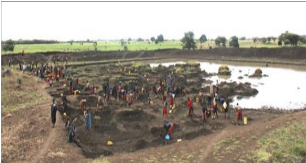
Construction of an excavated cum-embankment type valley tank by a local community in the Kotido District of the Karamoja Region
