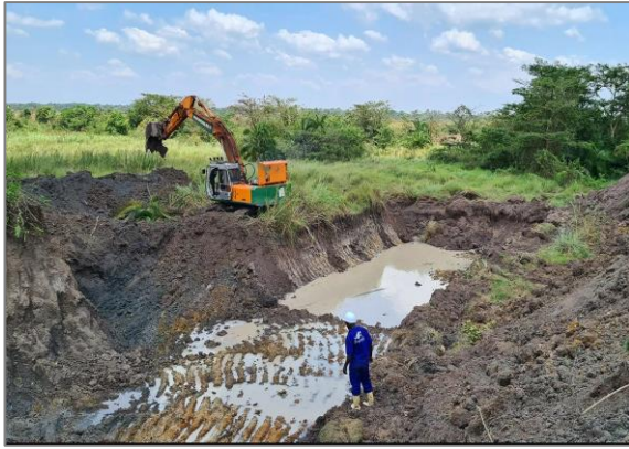
Construction of an excavated valley tank in hydromorphic grasslands in fat terrain
