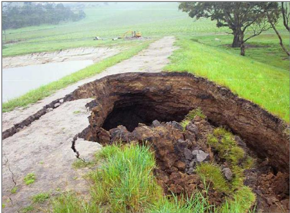
Failure of the wall of a small dam
