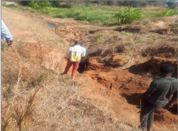
Extensive erosion of the downstream embankment and foot-slopes of a small dam
