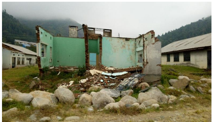
Figure 4-4: Some of the affected structures during the 2013 floods in Kilembe Subcounty
