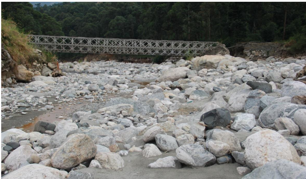
Figure 5-20: Broken bridges in kilembe destroyed by floods
