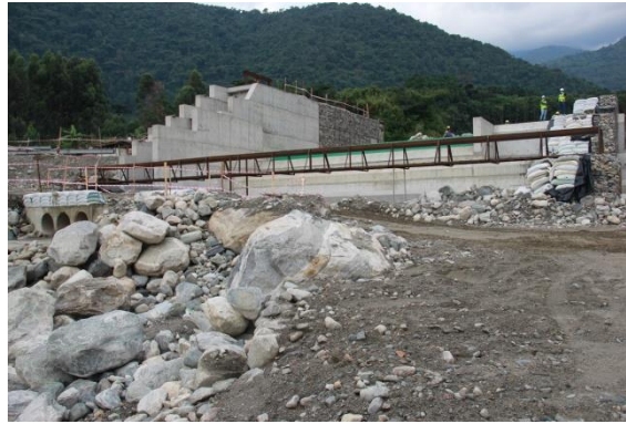
Figure 5-26: Nyamwamba II Hydro-power intake at risk
