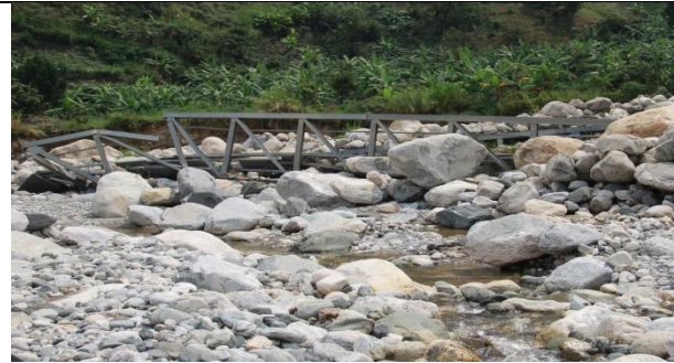
Figure 5-22: Damaged bridge between Kilembe and Maize factory
