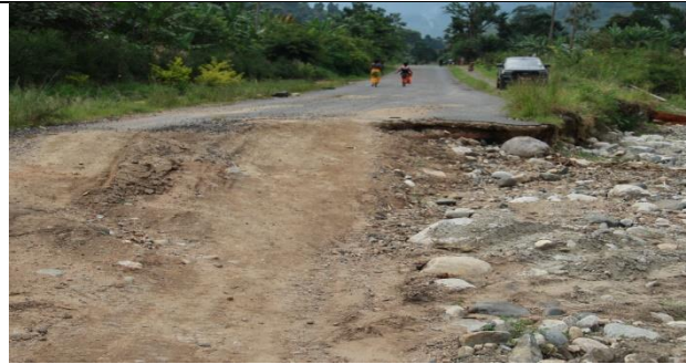
Figure 5-21: Damaged kilembe- Kasese town road
