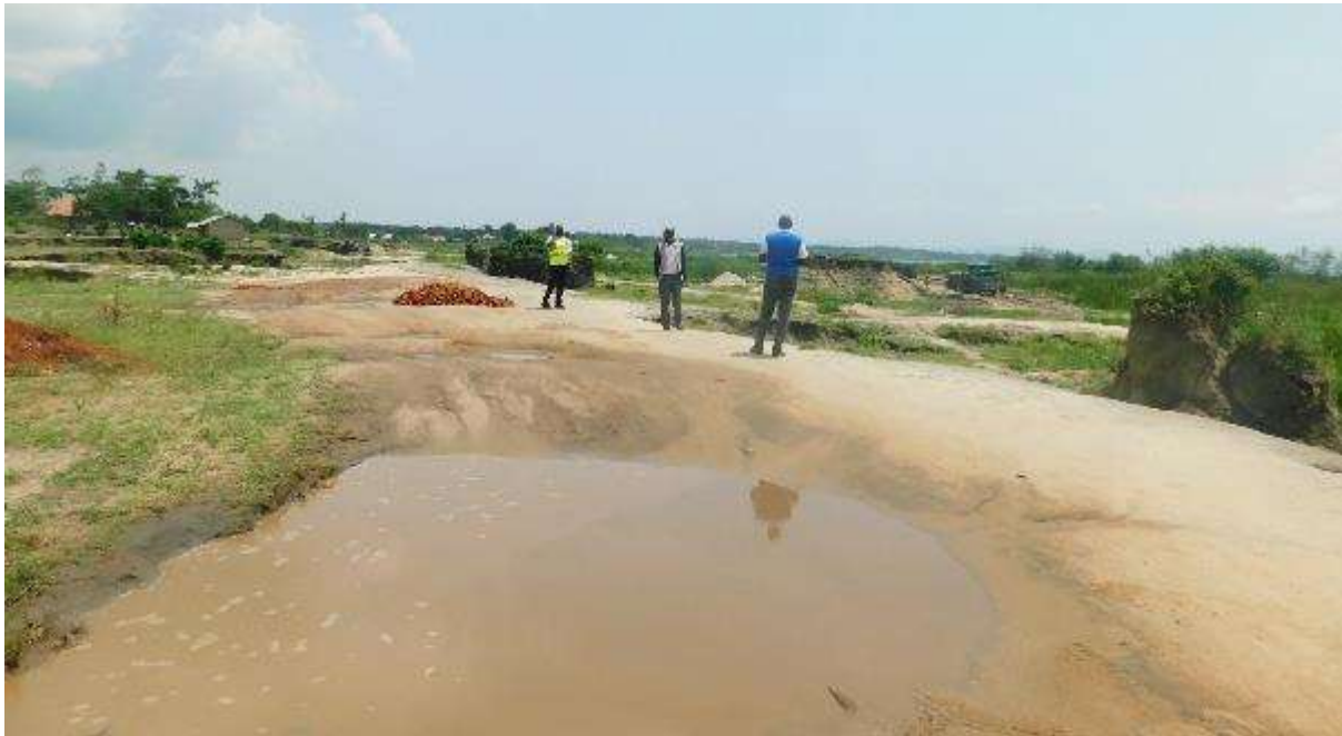
Figure 2-10: Part of the Access Road to the intake and WTP sites in Lugala Beach Village
