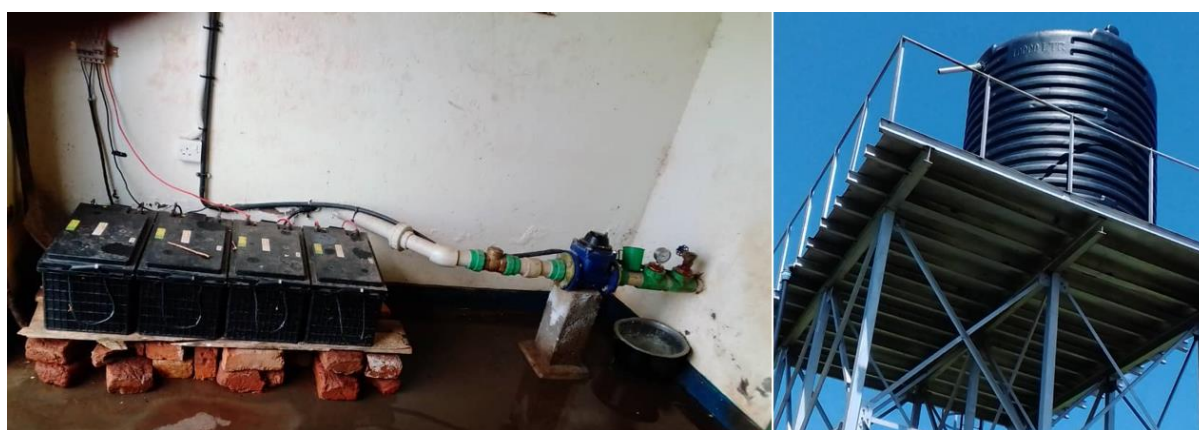
Figure 5-63: Current state of storage batteries and reservoir
