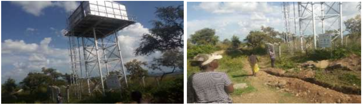
Figure 1-6 : Existing tank at Invempi Refugee Settlement in Nyaranga Village
