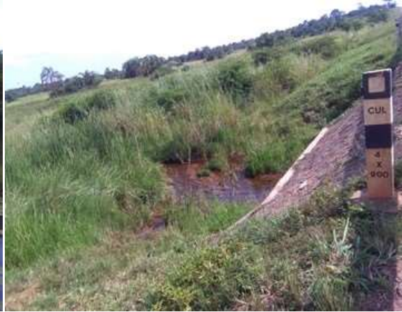
Photo 4: Extent of Water Level fluctuation in some waterlogged areas
