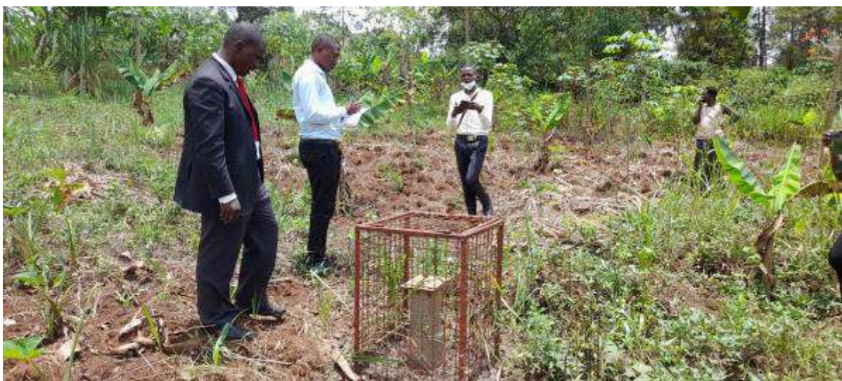
Plate 5: Kabamba water supply production well.
