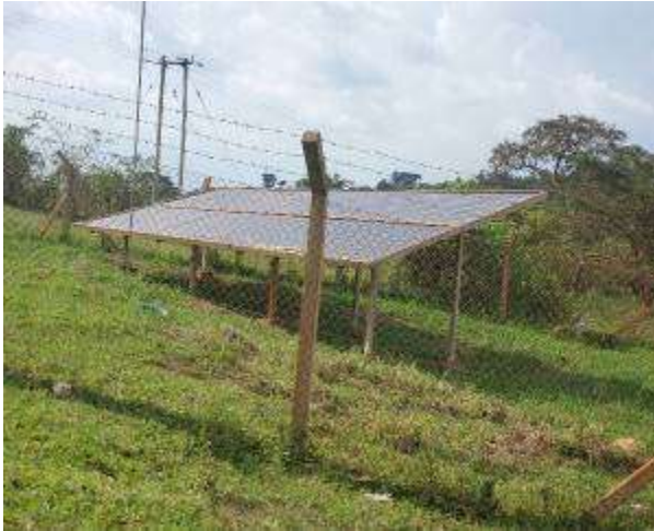
The source with a solar panels to enable pumping
