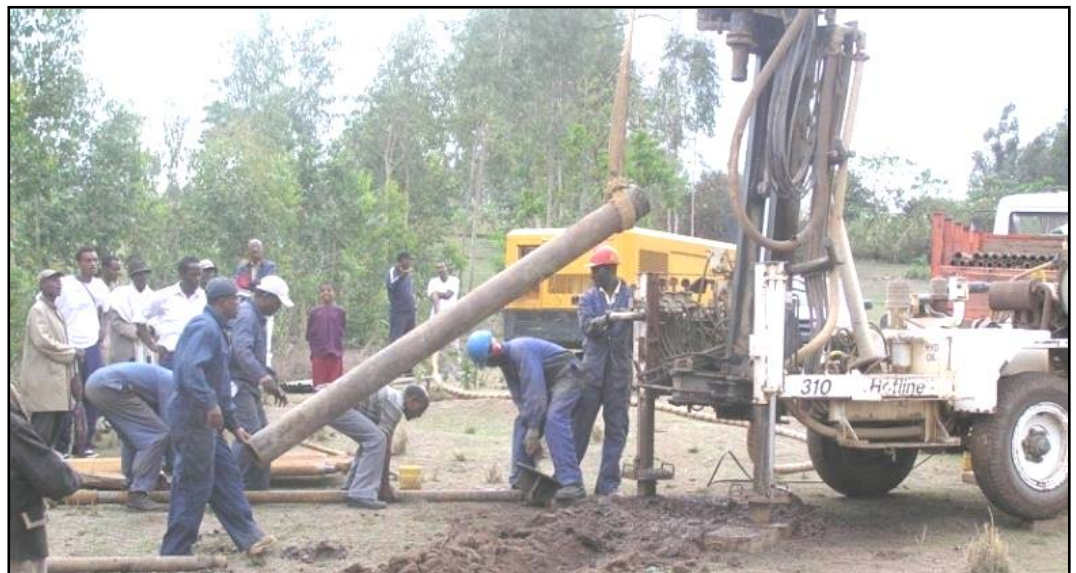
Figure 9: Poor Safety – No Hard Hat – No Clearly Defined Barrier
