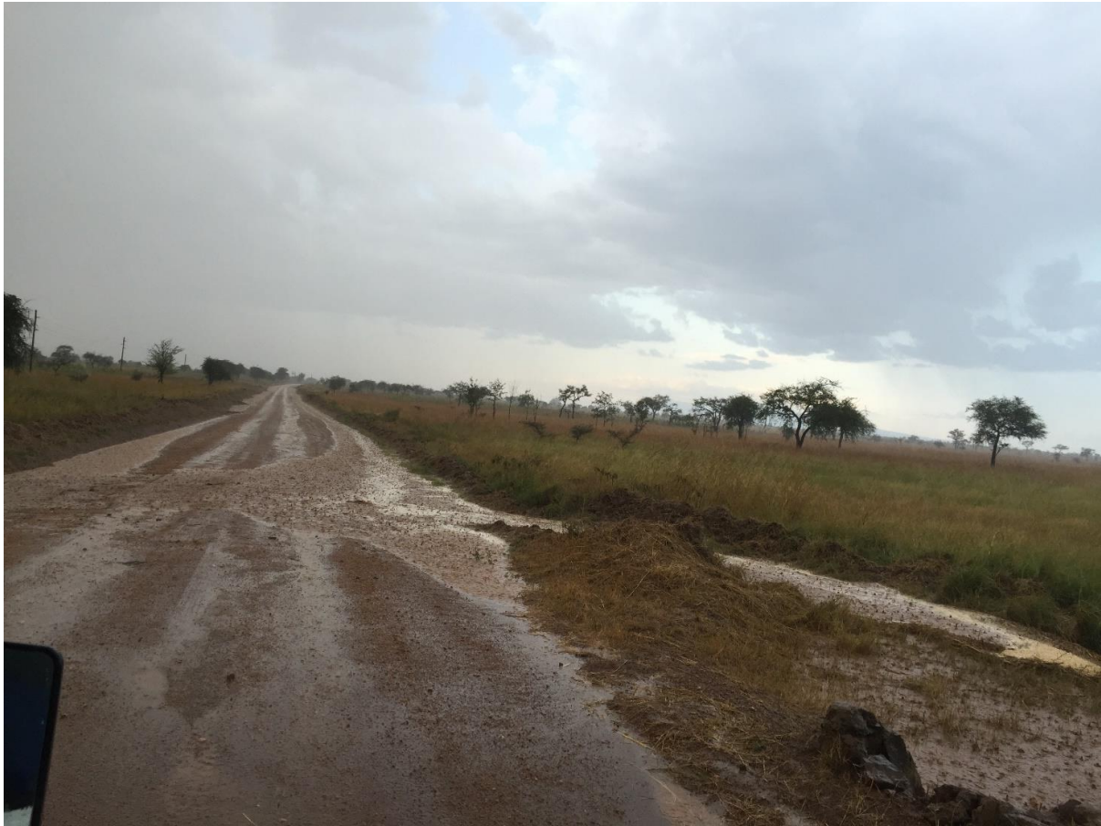
Figure 41: Road near Arecek Dam during the rain. Roads transport a lot of water that could be turned to good use.
