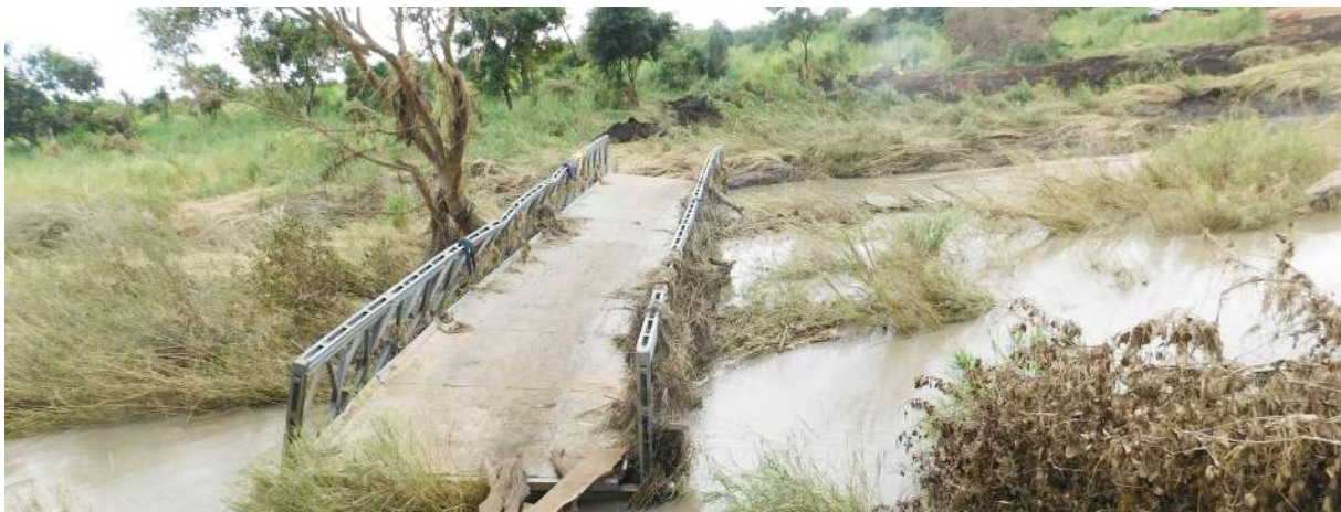
Bridge washed away by a flood in Unyama subcatchment in the Albert Nile
