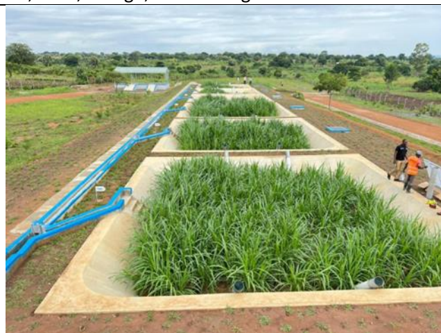
Photo 2: sludge drying beds for sludge treatment at Yumbe FSTP
