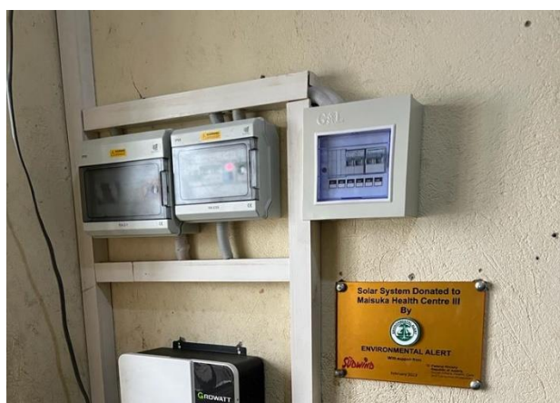
Photo 8.1.2: A hybrid solar system installed at Kyakahazire sub-county.
