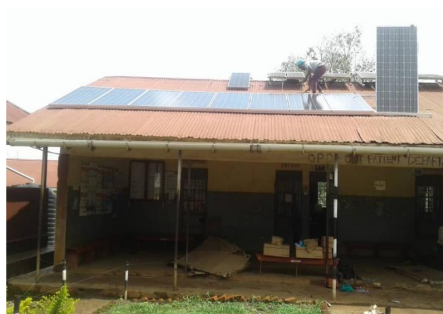
Photo 8.2.2: Solar panels on top of the Kyakahazire sub-county.
