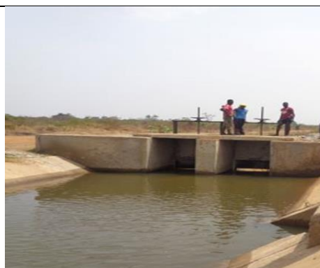
Photo 7.2-2: Installation of sluice gate at cross regulator 1 at Wadelai Irrigation scheme in Pakwach District
