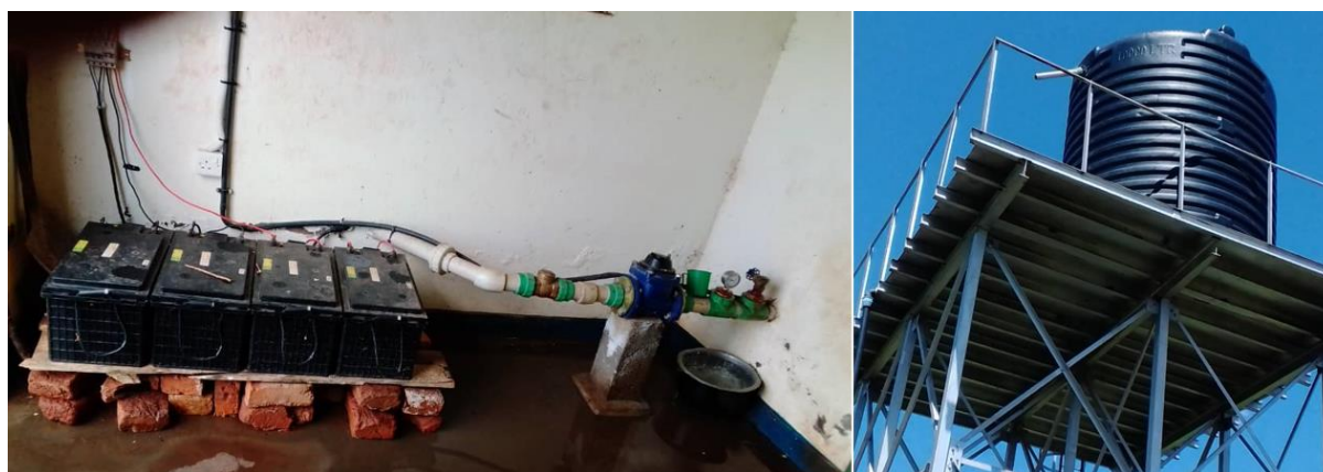
Figure 5-63: Current state of storage batteries and reservoir
