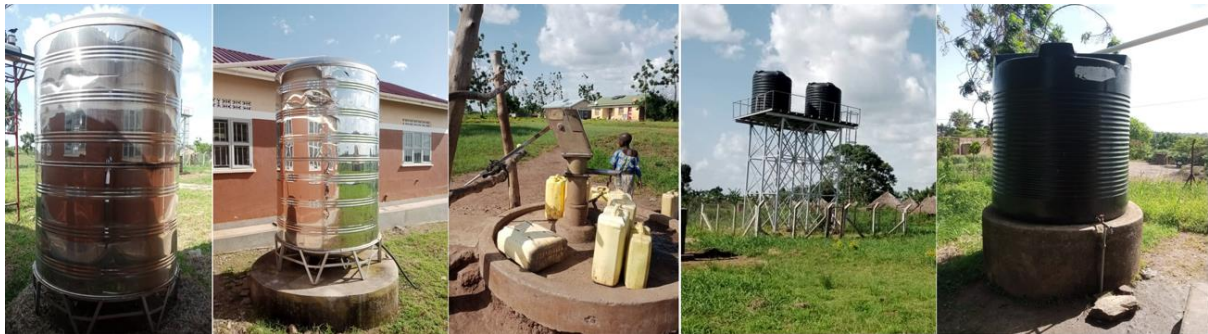
Figure 5-69: RWHTs, Borehole, Storage tanks at Apodorwa HC III with support from OPM/DRDIP/ World Bank
