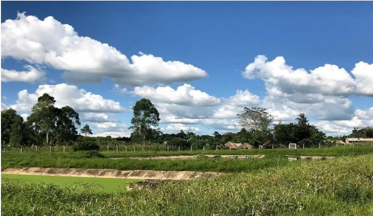
Figure 0-3: Waste Stabilization Ponds at Kiryandongo Hospital
