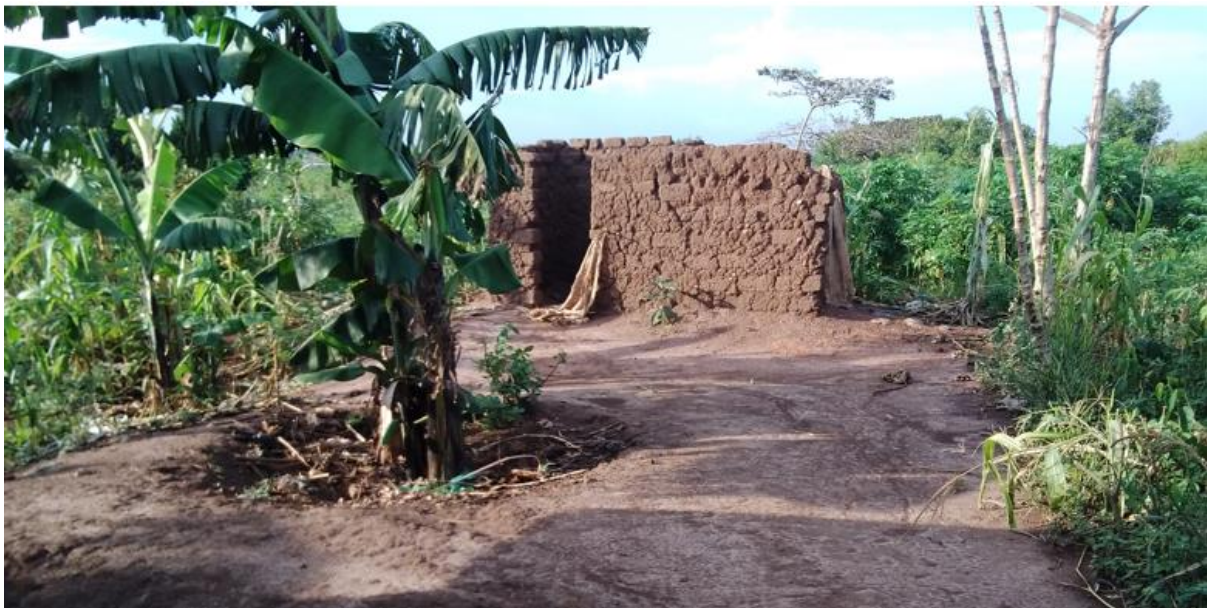
Figure 0-73: Poor pit latrine in Mutunda RGC
