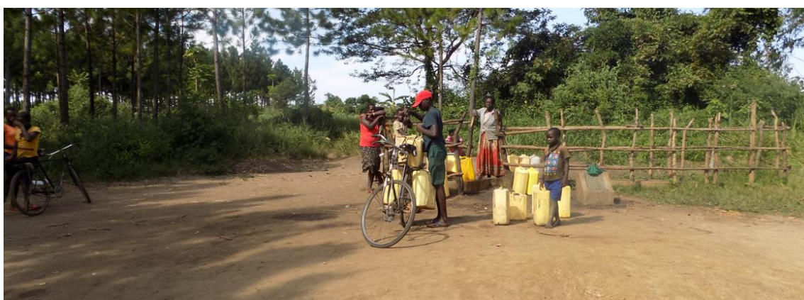
Figure 0-33: Community borehole (MGW1) in Popara West village - Mutunda sub-county
