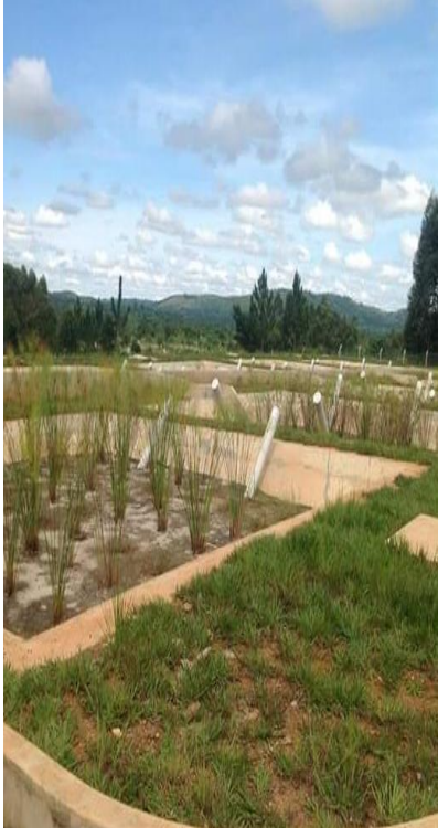
Fecal sludge treatment plant at Kasaali
