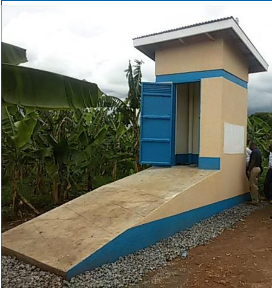
Household Eco-friendly toilet; One hundred eighty-eight (188) units were constructed for demonstration purpose.
