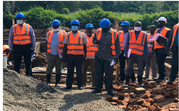
MWE Officials, project Staff together with the Contractor held a site inspection to assess the progress of the on-going construction works while maintaining COVID19-SOPs.
