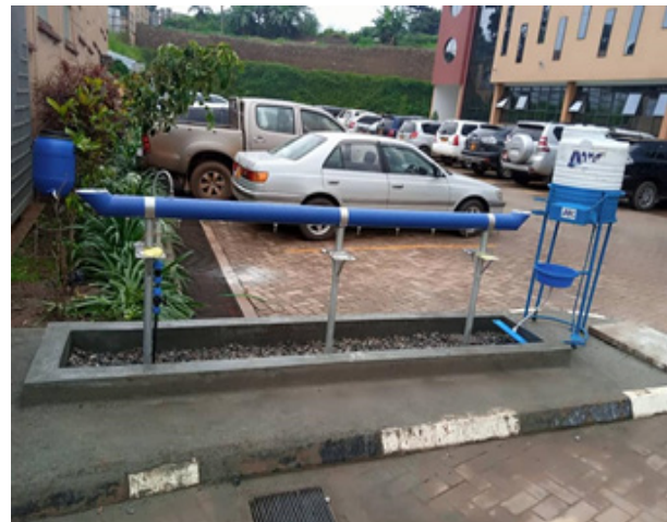
Sanitation measures and installed facilities at the Ministry Headquarters in Luzira to prevent the spread of COVID19 pandemic.
