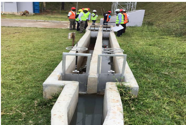
Inspecting the Shuuku-Masyoro Gravity Flow scheme at Sheema district aimed at increasing access to safe water, improving sanitation and hygiene
