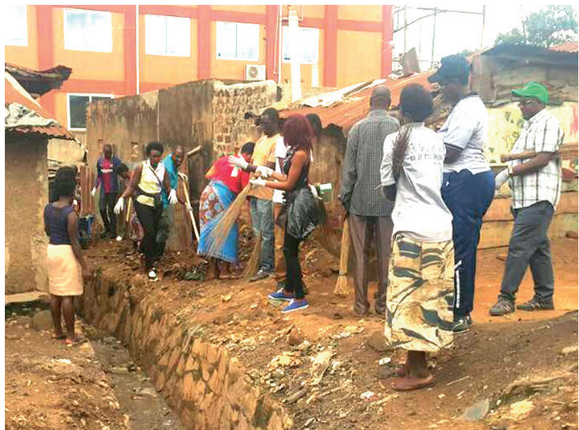
^^^^Sanitation clean up exercise at Kagugube at Makerere Kivulu during the start of UWEWK2018
