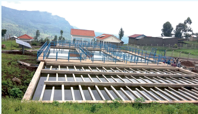
^^^The Lirima Treatment Plant in Manafwa District
