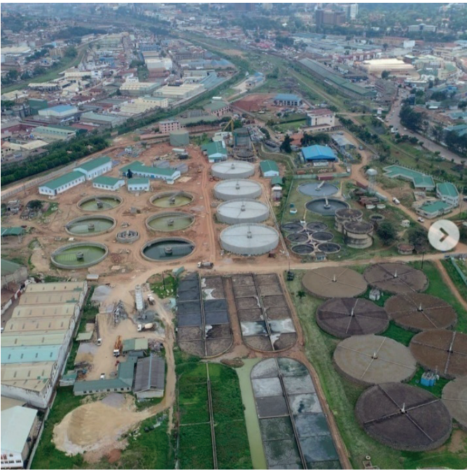
NWSC is constructing the largest sewage treatment plant in East Africa and Central. The plant when completed will improve sanitation of over 850,000 city dwellers in Kampala.
