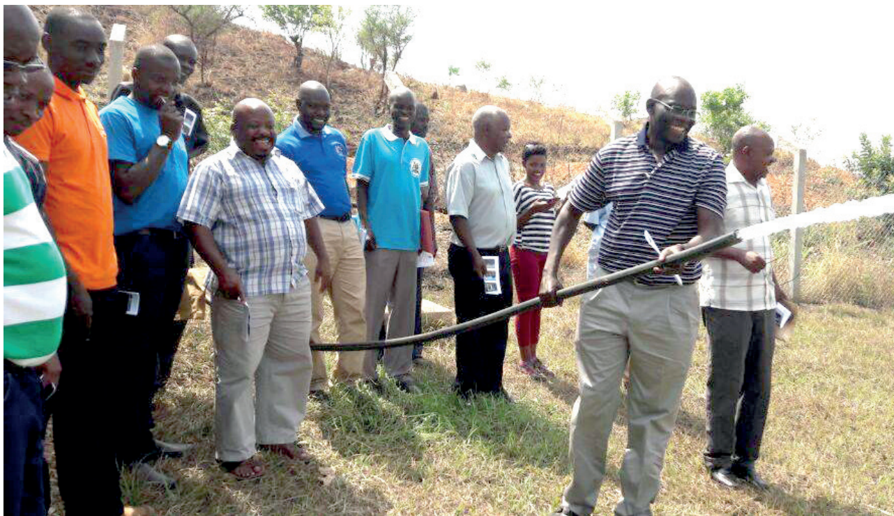
^^^ Rural Water Supply and Sanitation Department testing the water pressure during the technical commissioning of the Wadelai Water Supply and Sanitation system
