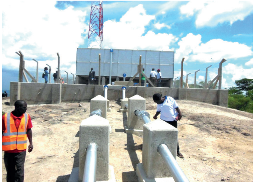
^^^A 150 cubic meter cold pressed steel tank for the Kakumiro Water supply and sanitation system in Kibaale district.
