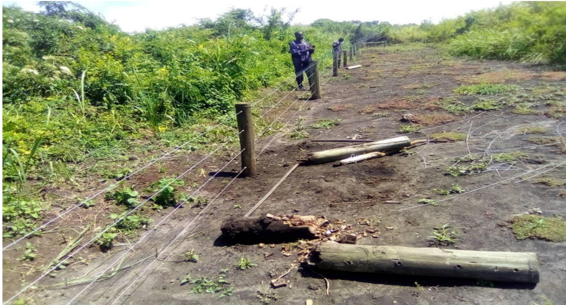
Figure 24: Examples of gum fence poles being replaced at QECA at the moment
