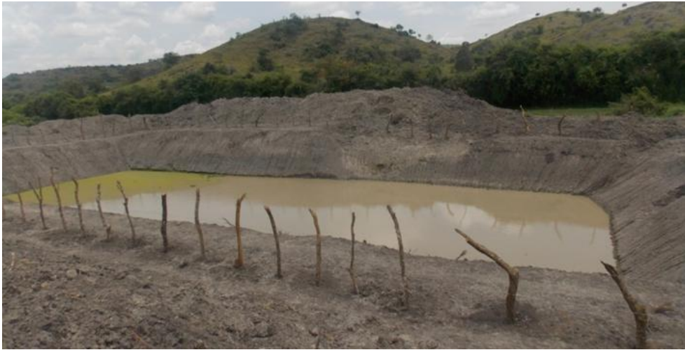
Figure 12: Akayanja water valley dam constructed using revenue sharing funds in Lake Mbuoro NP
