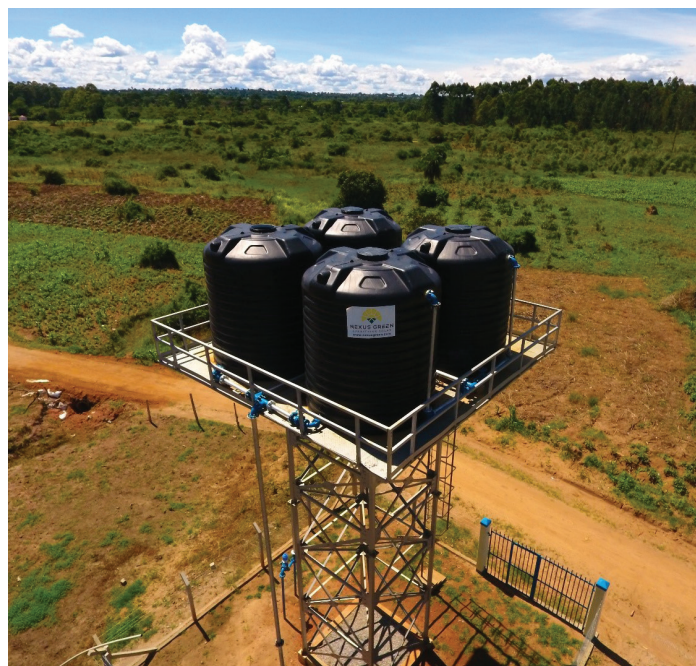
Reservoir tanks supply water to the gardens
