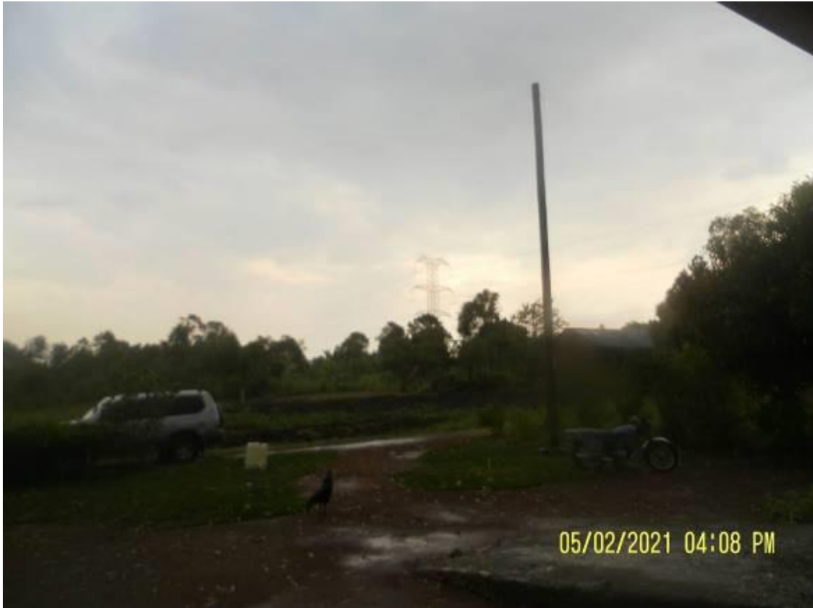
Figure 4-4: Electricity line under construction at Mr. Patrick Ogwok’s home from which the Kigumba Faecal Sludge management facility site can tap
