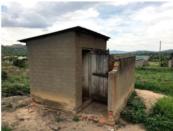
Unlined Pit Latrine at Kyalulangira Sub – County Offices
