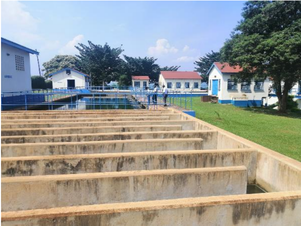
Plate 4.24: The clarifiers for the existing treatment works
