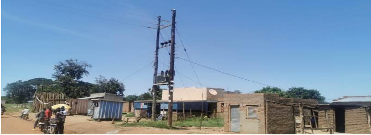
Plate 11: Transformer in Barr trading Centre
