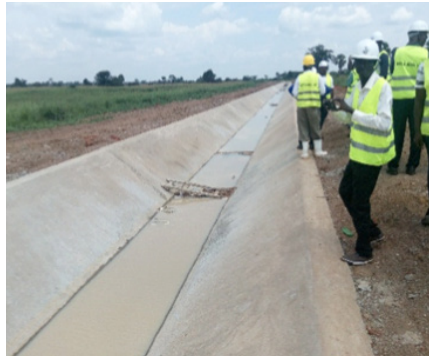
Completed concrete lining of main canal at Doho II irrigation scheme, Butaleja district
