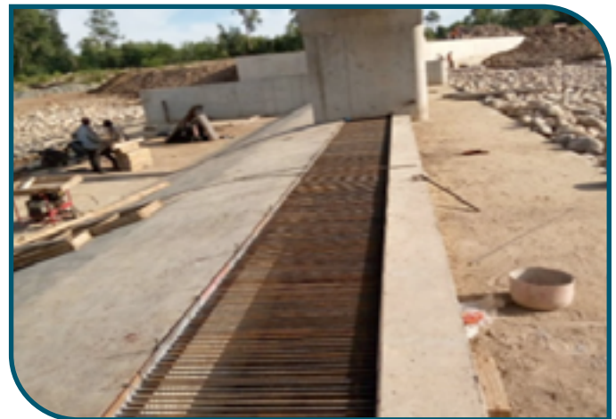
Placement of the trash rack along the weir channel at Mubuku II irrigation scheme, Kasese district ■
