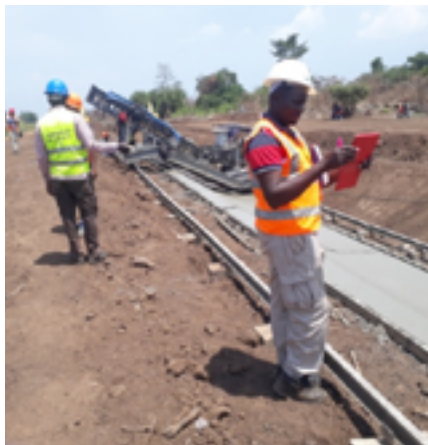
Canal construction using a concrete paver at Wadelai Irrigation Scheme, Pakwach district ■
