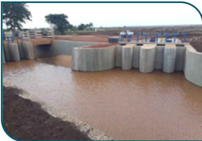
Completed head works on River Kabajiria at Ngenge irrigation scheme, Kween district ■
