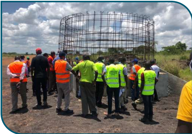
Project steering committee inspecting work at the dry well that will form a control point of flow through the intake at Wadelai irrigation scheme ■
