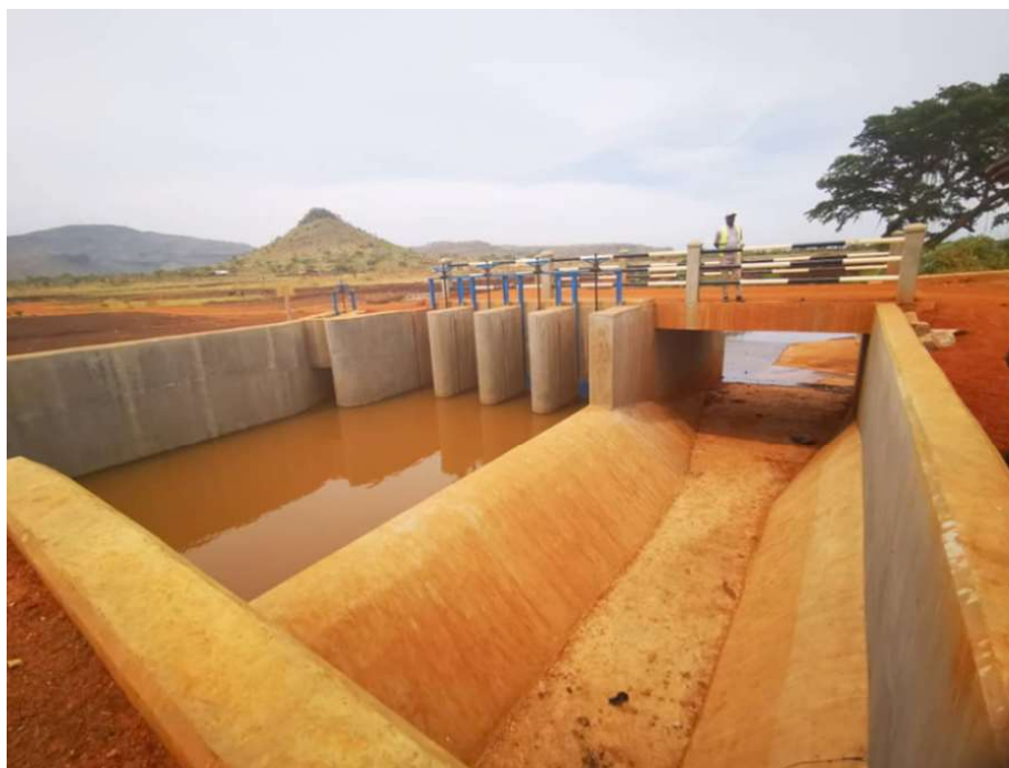
A view of the upstream side of the Head works before flooding■
