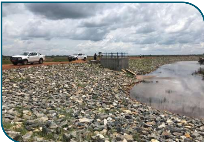
An upstream side of a protected embankment with riprap at Tochi irrigation scheme, Oyam district ■
