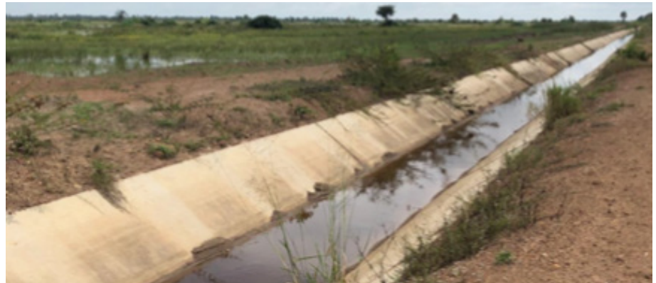
Concrete lining of the main canal at Wadelai irrigation scheme, Pakwach district ■
