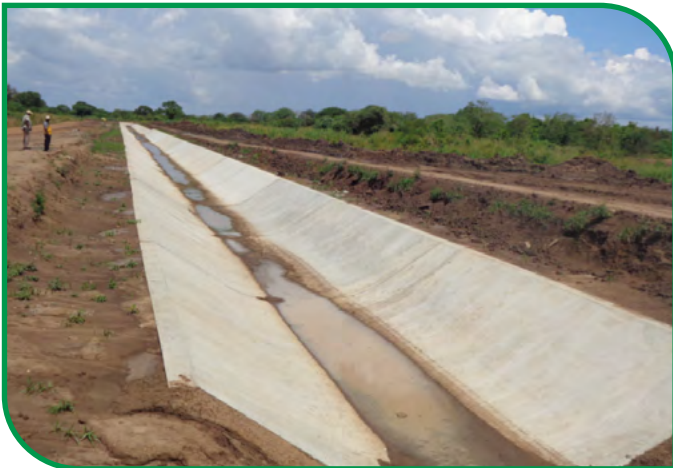
One of five secondary canals under construction at Wadelai irrigation scheme in Pakwach district ■
