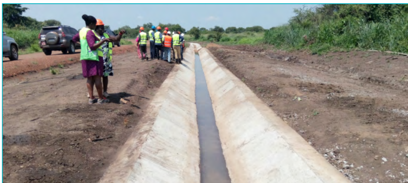
One of the secondary canals completed at Wadelai irrigation scheme, Pakwach district ■
