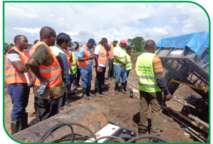
Members of FIEFOC 2 Project Steering Committee inspecting ongoing construction work of canals using advance machines at Wadelai irrigation scheme, Pakwach district ■
