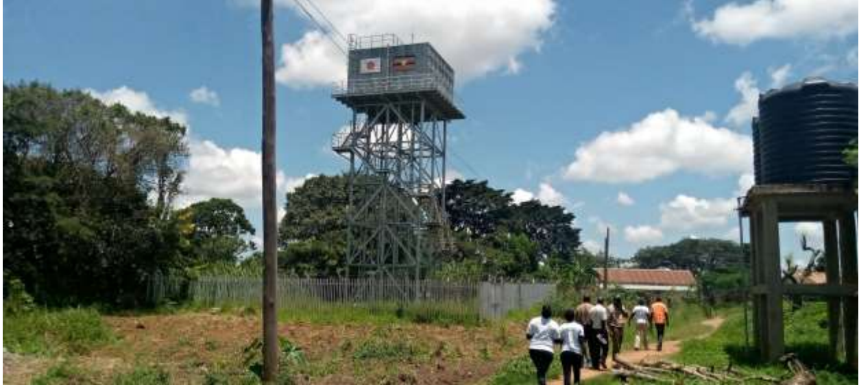
Figure 2-15: Showing one of the existing water reservoir/ tank at Kidetok Girls SS which will be used as the supply point for Kidetok Town Council.
